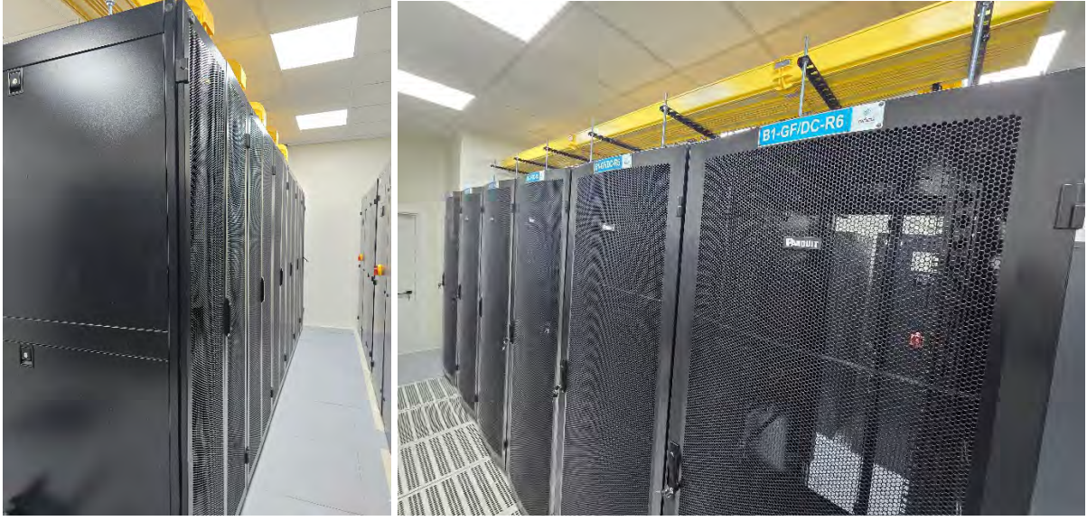
TAHAKOM HEAD OFFICE Riyadh (DATA CENTER)
