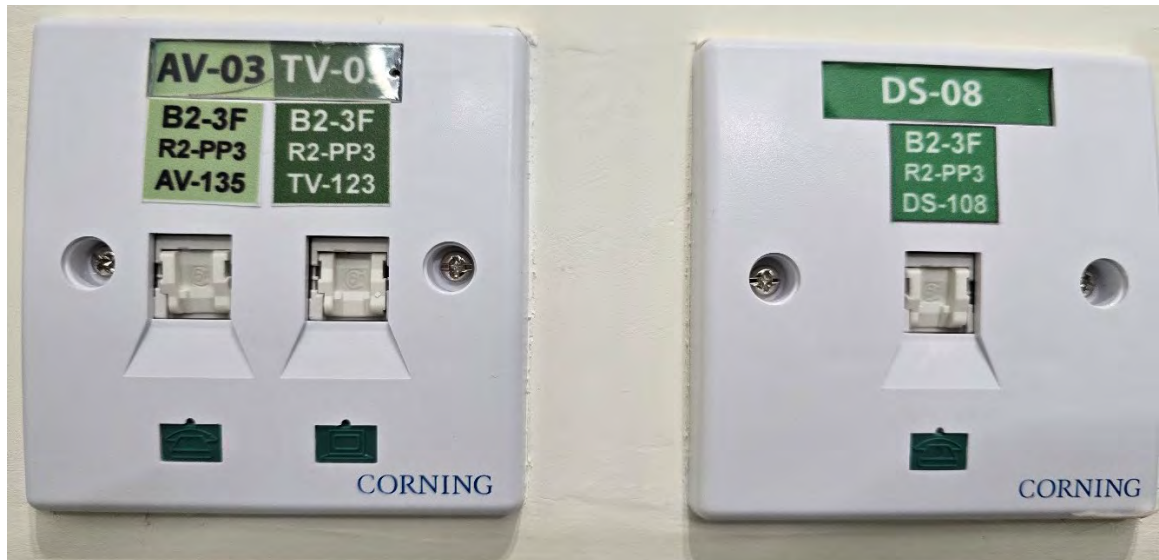
TAHAKOM HEAD OFFICE Riyadh (User Side Face Plates)
