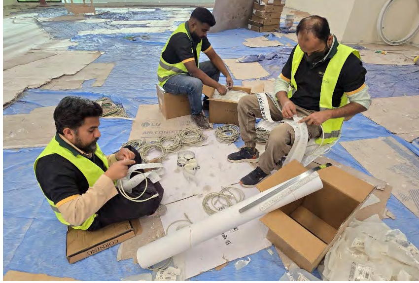
TAHAKOM HEAD OFFICE Riyadh (Patch Cord Labelling)
