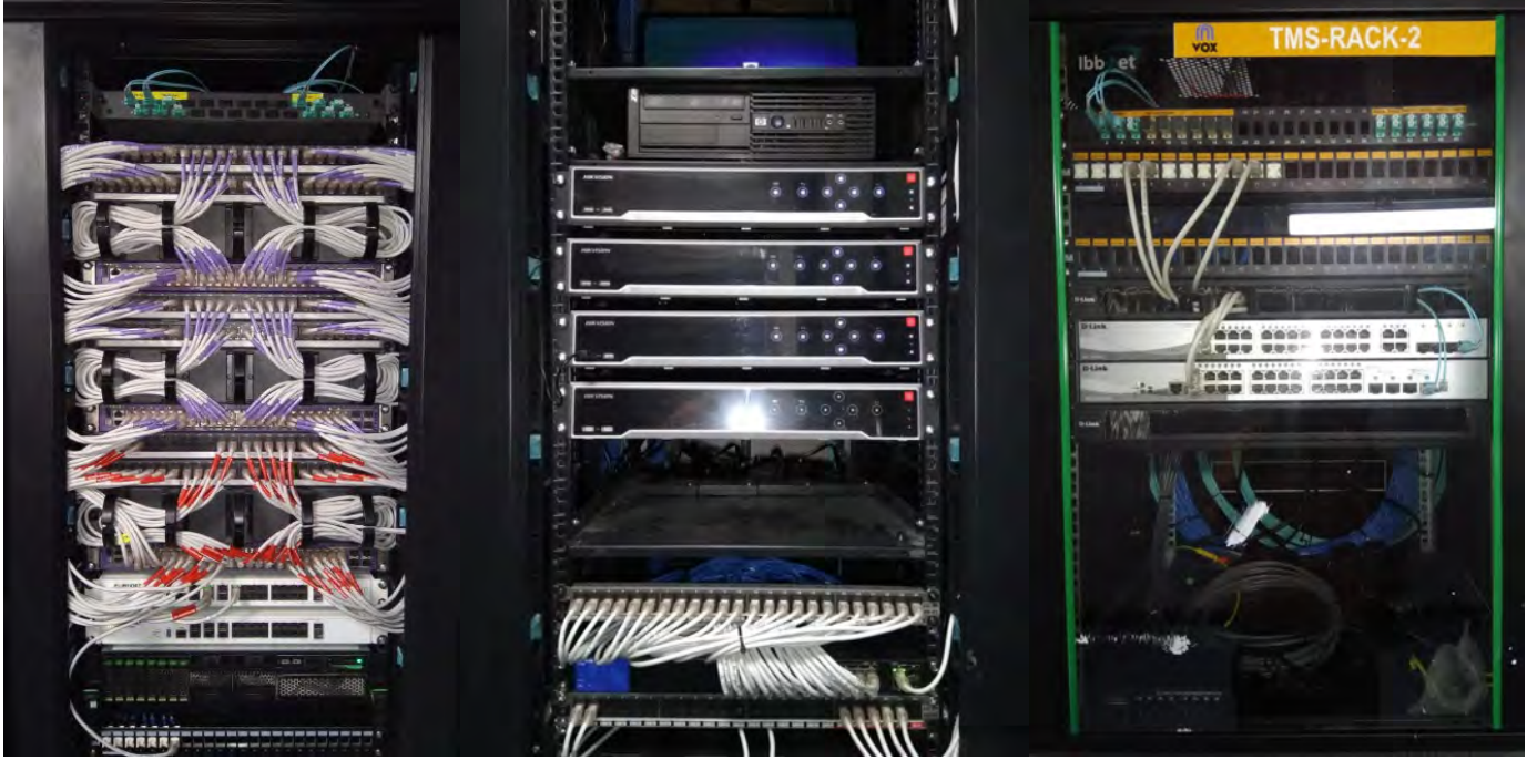
VOX Cinema Riyadh Front, Riyadh. (Data Center)
